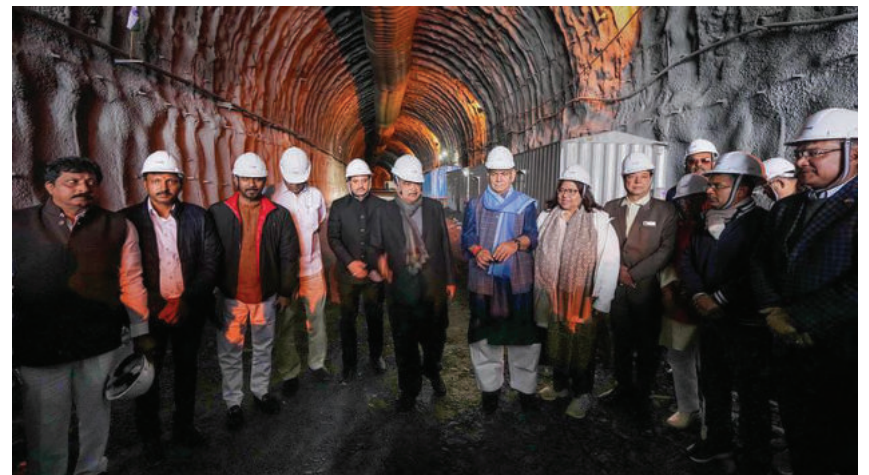
All-weather link: Union Minister Nitin Gadkari, along with J&K Lt. Governor Manoj Sinha, inspecting the tunnel work in Ganderbal. PTI
